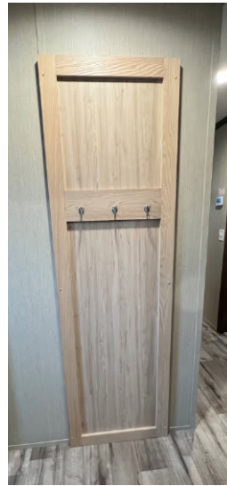
Coat Rack Water Heater Access Panel
